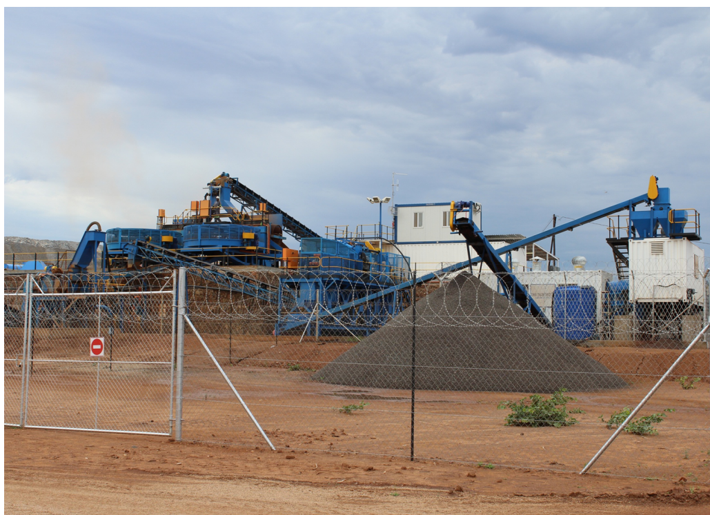
Figure 9: Image of the 200t/h modular processing plant.
